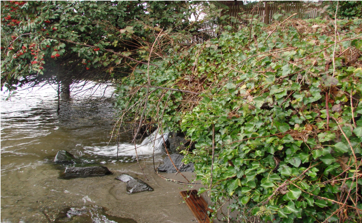
Photo #9 – Outfall into Lake Washington – viewing north along shoreline
